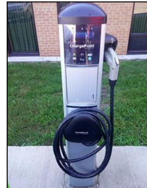
Electric car charging station Source: www.choosecornwall.ca
