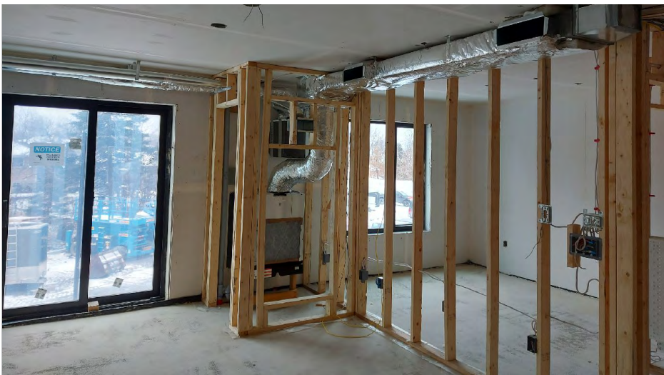
Heat pumps have been installed in every unit in this City of Cornwall affordable housing development.
