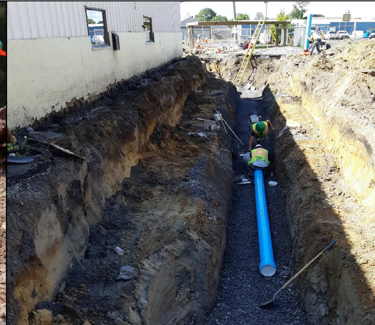
As part of the site servicing of the MW Yard a new 200mm diameter PVC watermain was extended from St. Michel Ave. easterly to service both existing and future buildings.
