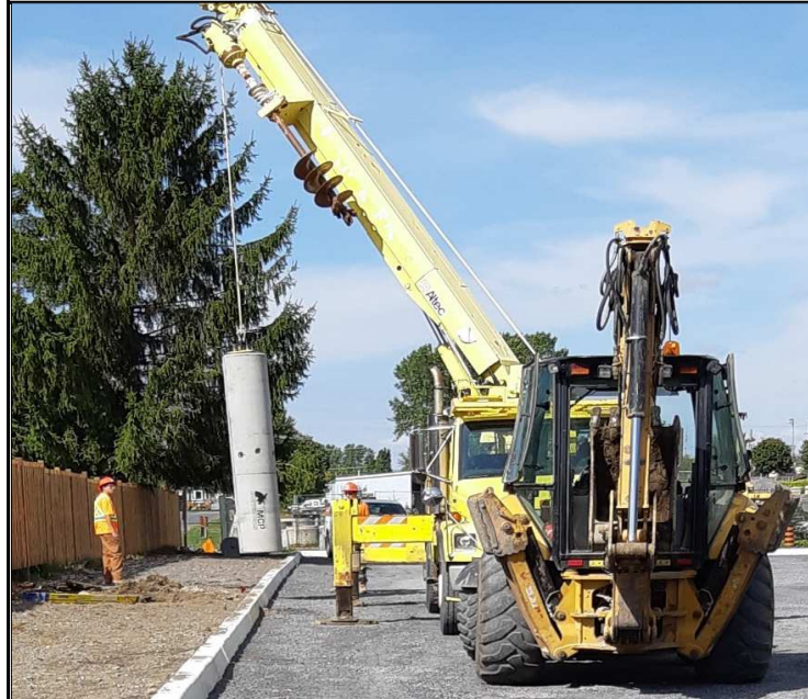
As part of the construction of the new parking lot located on Twelfth St. new light standards with concrete bases (as seen above) were installed.
