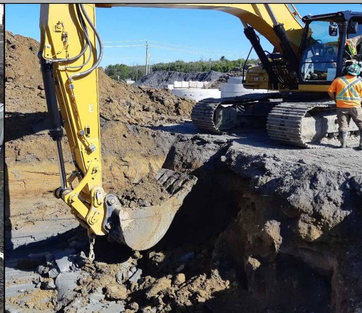
During excavation the Contractor encountered a wet gray clay (see bottom left corner) that was removed and could not be reused as the material is not considered suitable for backfill or as a base for building.
