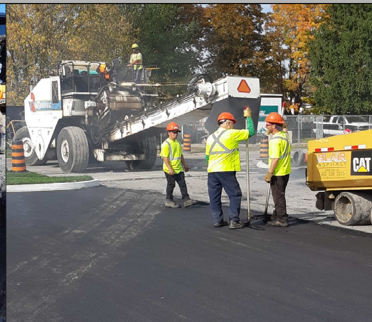
As part of the work included in 2019, the new parking lot on Twelfth St. was paved. Above is a photo of paving operations in progress.
