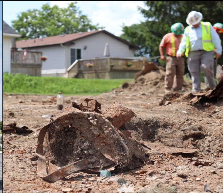
During excavation for the construction of the new parking lot, garbage/landfill material was encountered and required removal.
