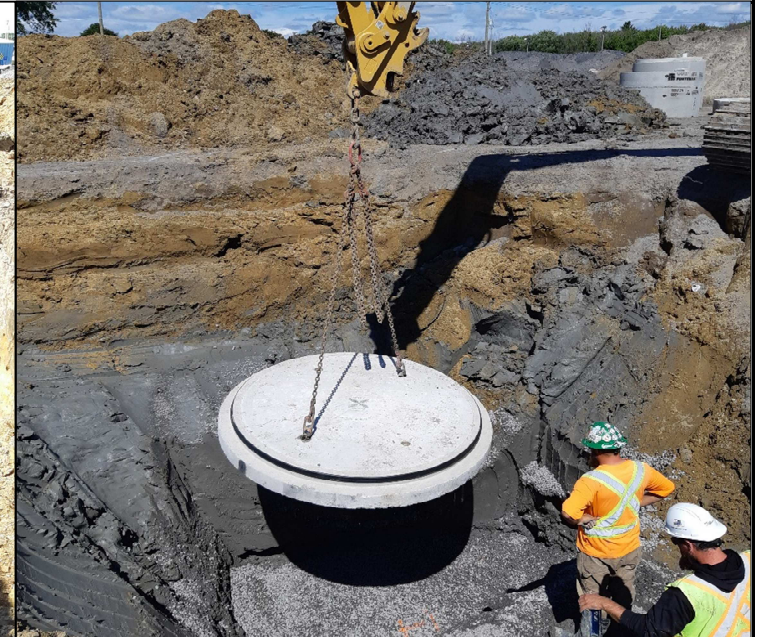
As part of the site servicing of the MW Yard an oil/grit separator was installed south of the fuel station to minimize the likelihood of any fuel/oil spills or grit resulting from operations flowing into the City's storm sewer network.
