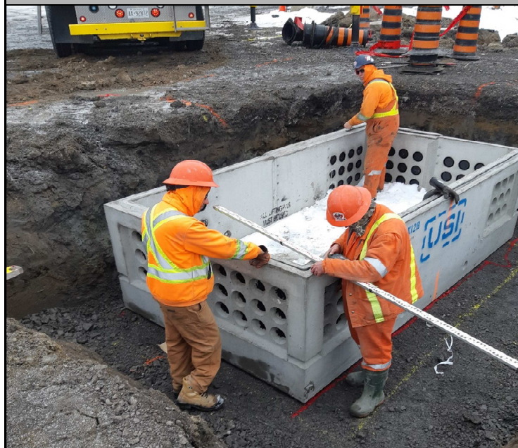
As part of the servicing for the MW Yard, a system of conduit for future electrical and communications services was constructed. Pictured above is an electrical maintenance hole which will provide access to the conduit.
