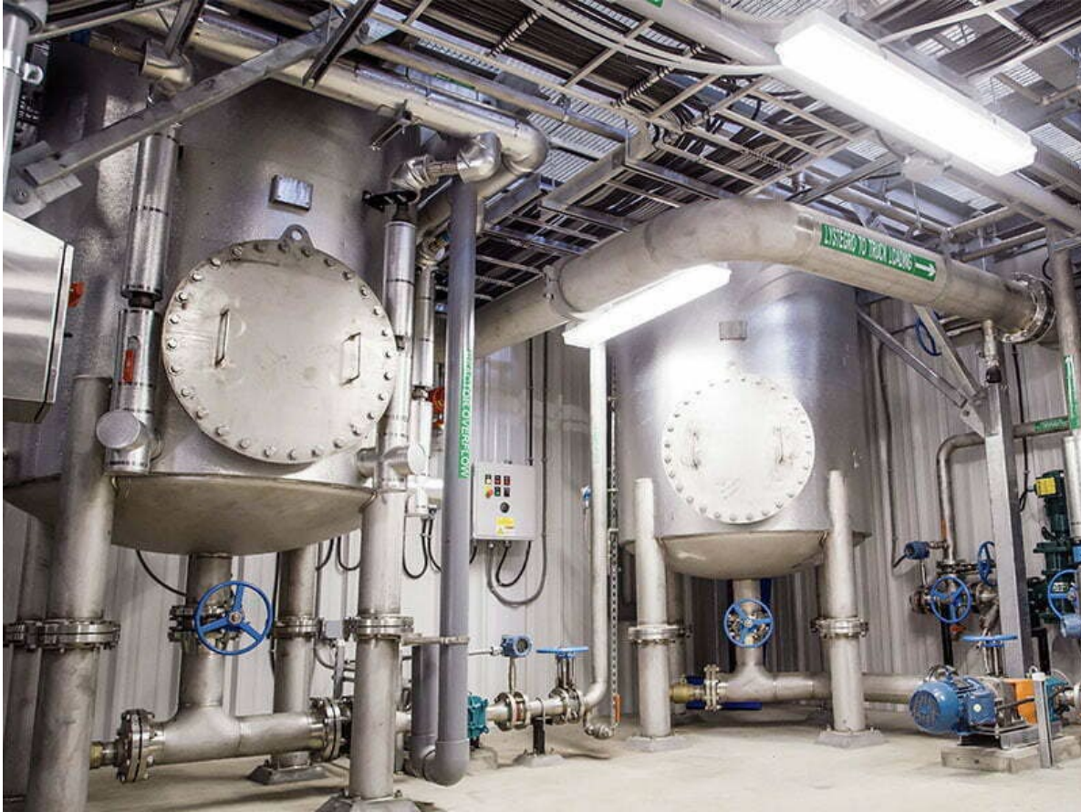
Figure 4.2 Example THP Reactors installed in-facility at Lakeshore WPCP in Innisfil, ON (Courtesy Lystek International)
